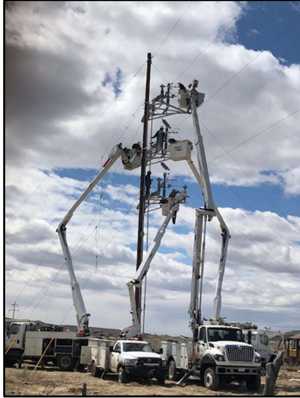
Figure 13. System upgrades on 69 kV switch
