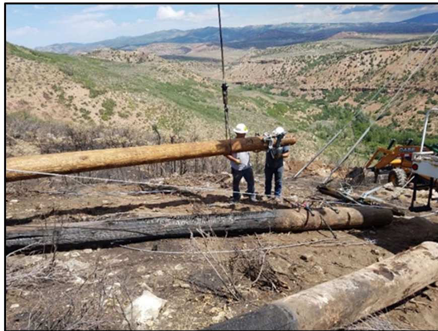
Figure 11. 3 Pole Structure damaged on Dollar Ridge fire of 2018.
